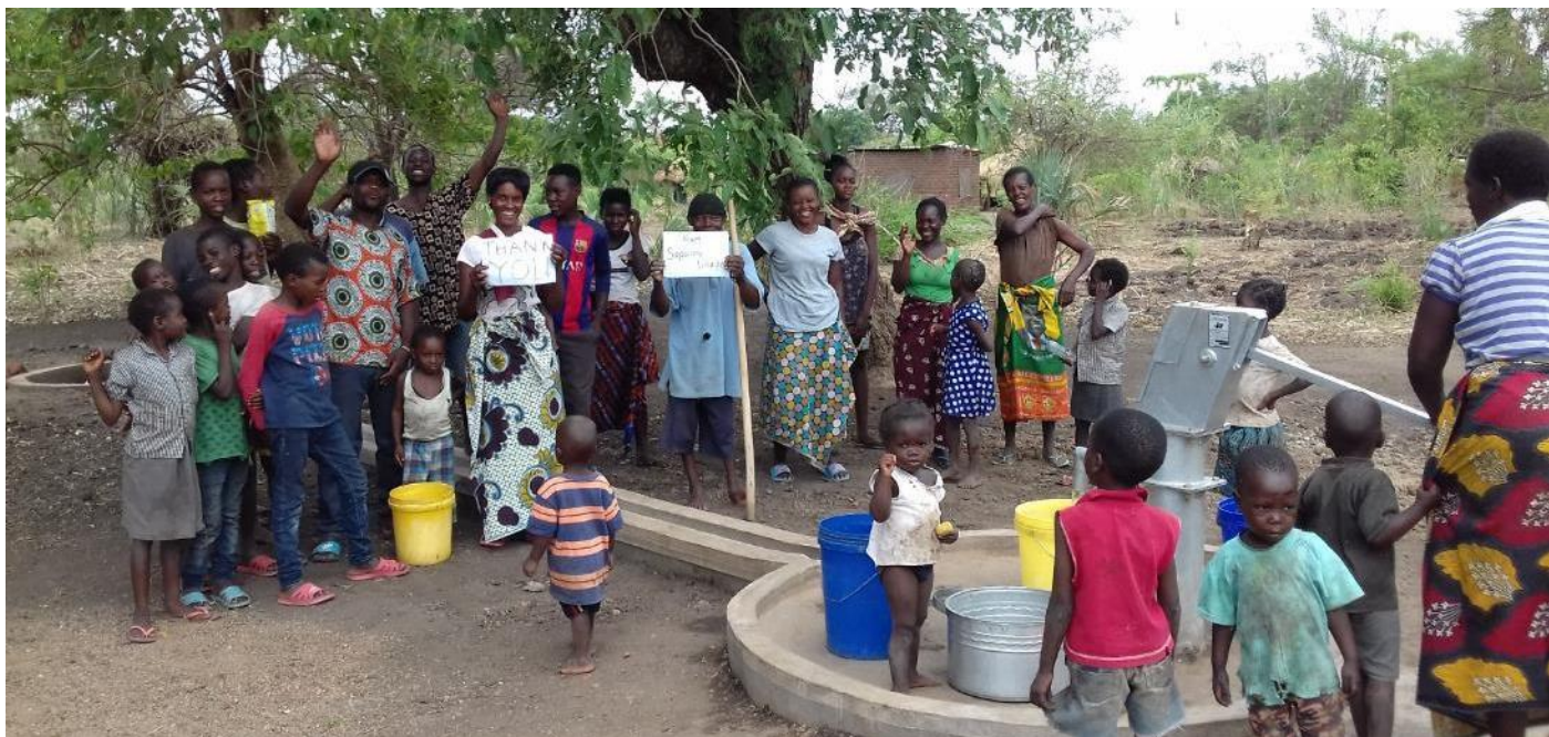
The new borehole at Sapulani shared with Zakeyo – thank you from the residents. Our unique ‘garden pond’ design. Residents use the overspill water from the borehole run off for vegetable gardens, domestic stock – chickens, ducks, goats – rather than the water just going to waste.
