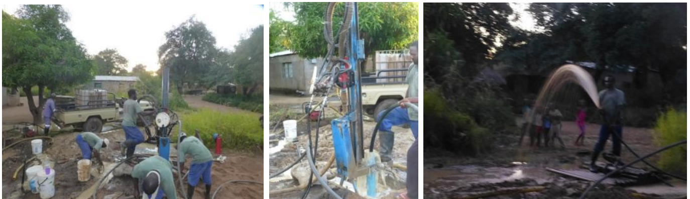
Drilling underway at Kopa Village. Pump testing was done quite late hence the poor quality picture!
