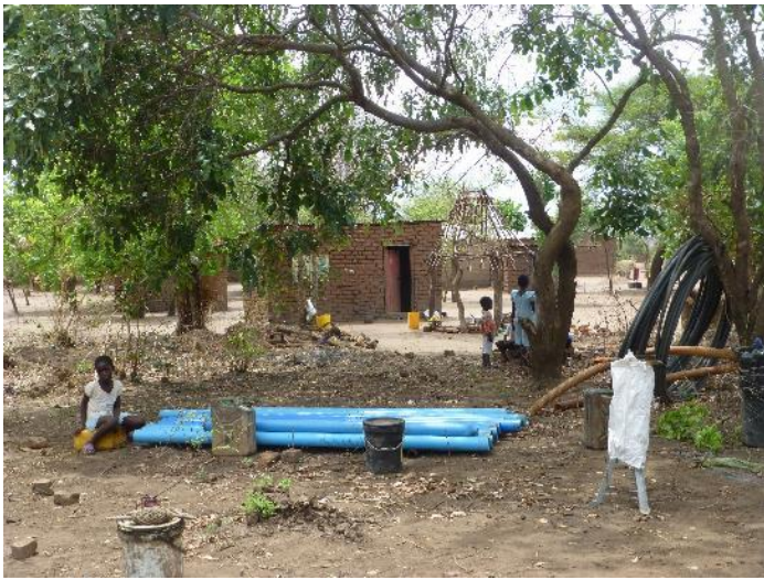
Some of the UPVC borehole casings 'under guard'
