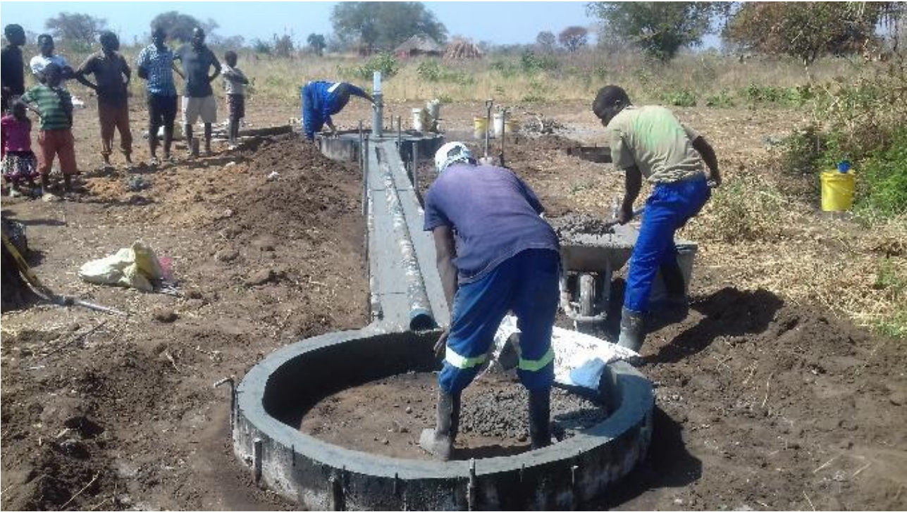
Headman and colleagues look on as the surrounds and garden pond are constructed.
