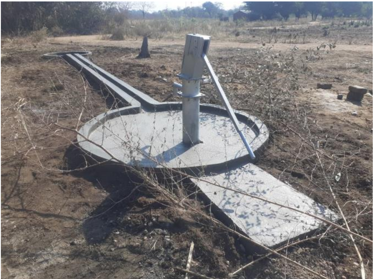
The finished borehole with handpump, surround, pumping platform, run off and garden pond. It must not be used for a few days in order for the concrete to set – hence the thorny branches temporarily protecting the works.
